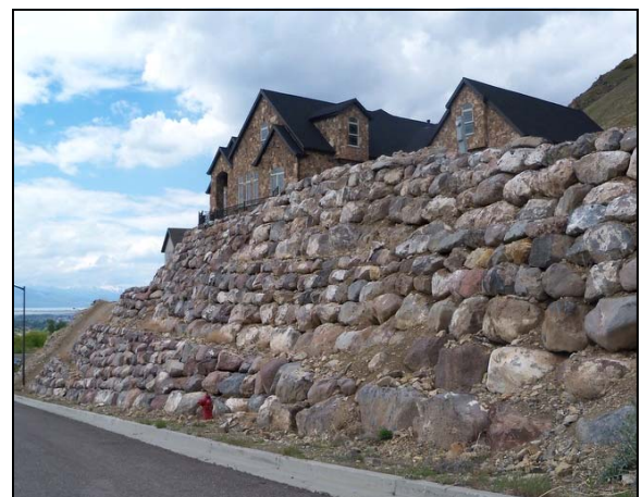
Figure 10-7 Excessive Hillside Development
